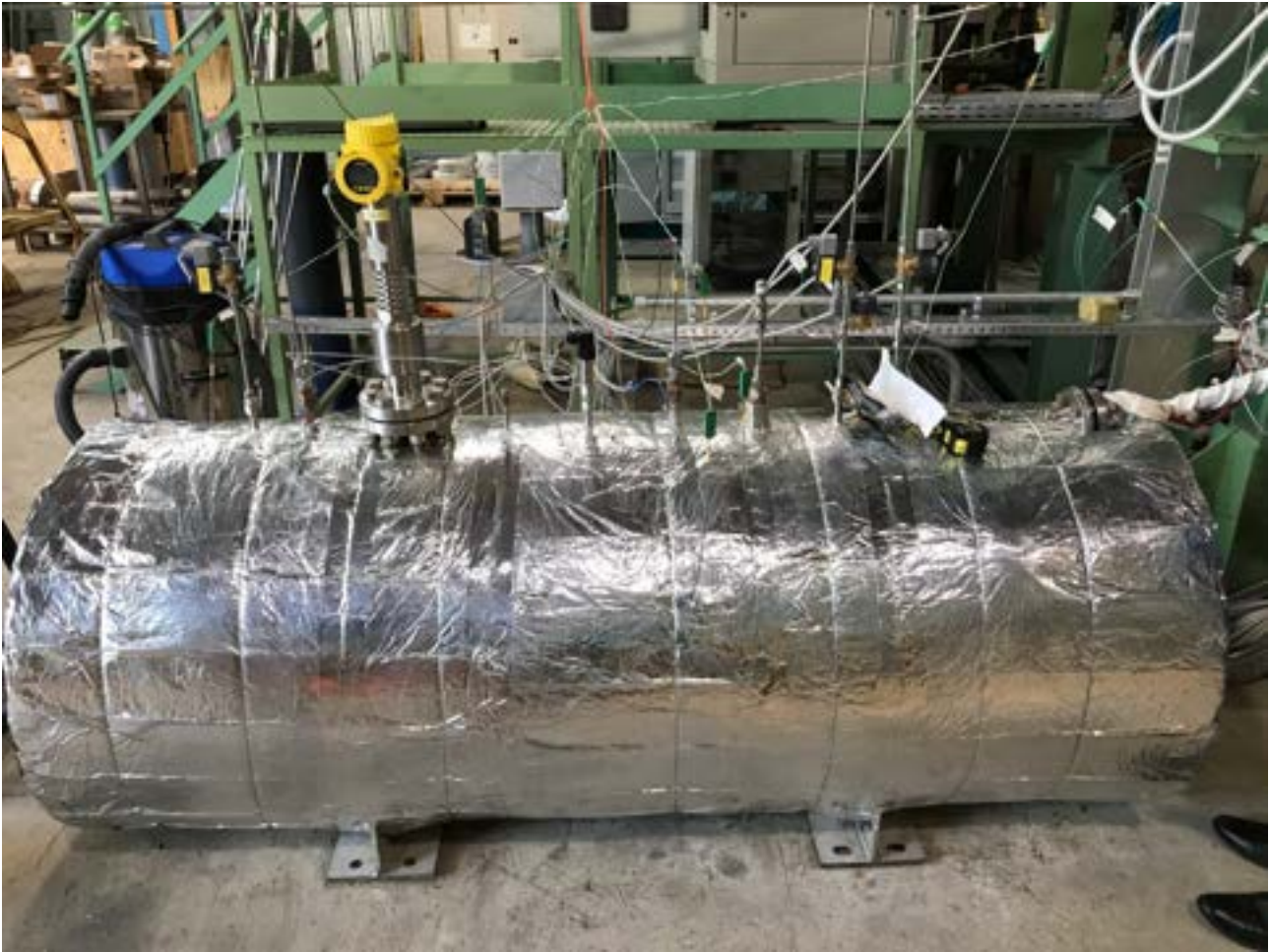
Fig. 2—5 – S4_A storage tank.
