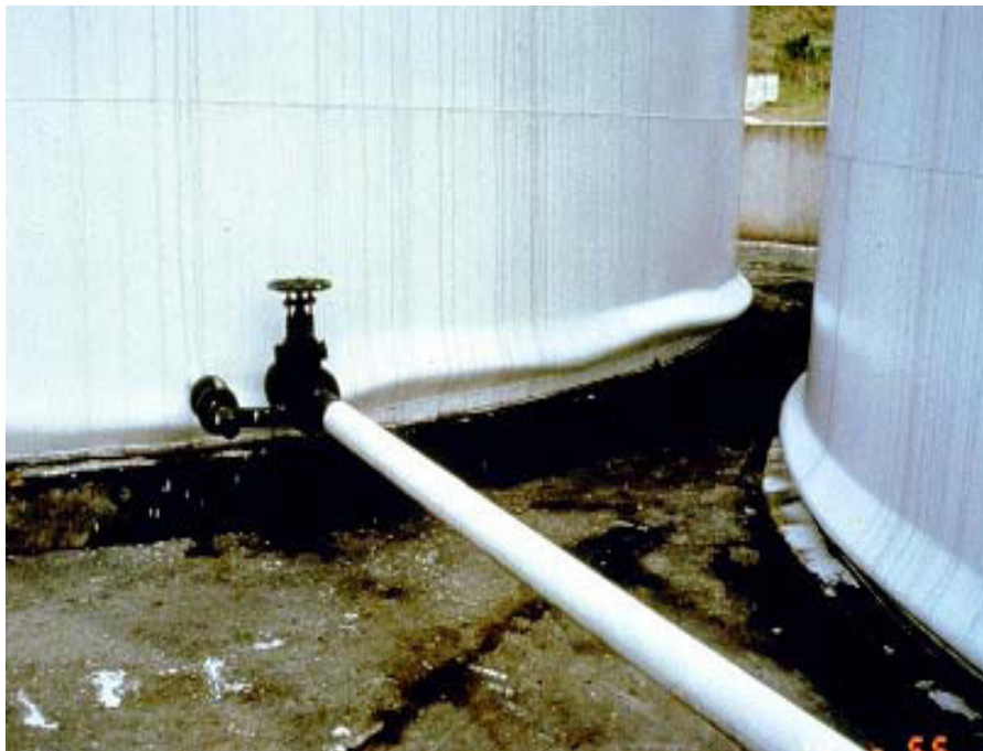
Figure 2 - Elephant's foot buckling deformation
