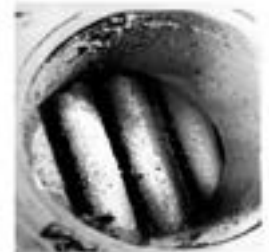
Slag deposit in heat exchanger
