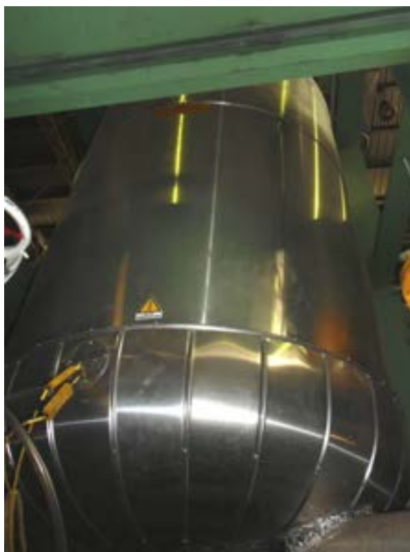
Fig. 9 – S3V dump tank.
