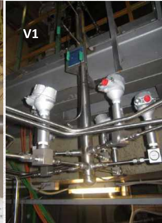
Isolation valve V1 Manifold 7 turbin flow meter
