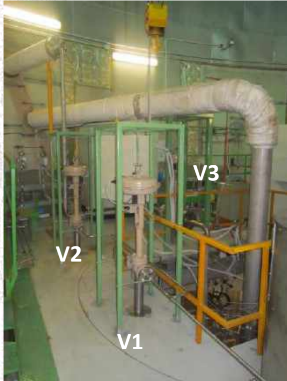
V1 isolation valve V2 bypass valve V3 regulation valve
