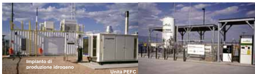
Energy station - Air Products/Plug Power (Las Vegas, NE, USA)
