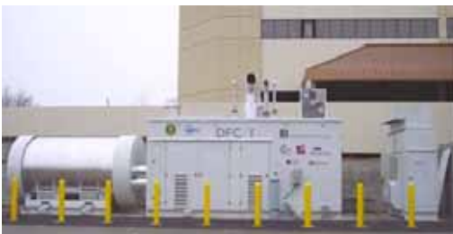
Impianto DFC/T®, Billings Clinic (MT, USA)
