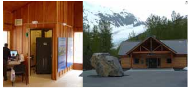
Sistema CHP da 5 kW (Exit Glacier National Park, Alaska)
