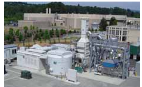
Impianto da 1 MW (DFC 1500, King County, WA)
