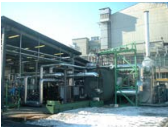
Figure 15. AFCo's Hybrid MCFC-GT installation in Milan (courtesy of CESI Ricerche)
