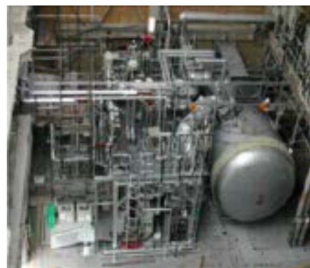
Figure 6. Full view of 300 kW class Compact System in Kawagoe Test Station
