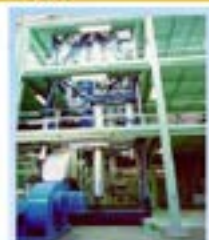
He-FUS3 Facility @ ENEA-Brasimone
