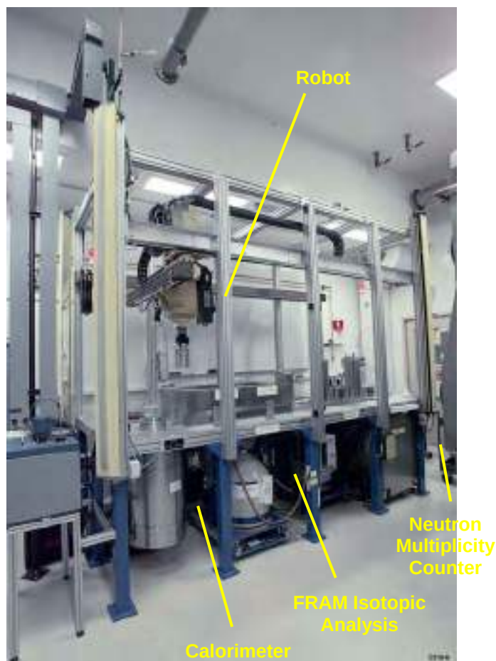
Fig. XIV-3. The ARIES NDA system installed at the Los Alamos Plutonium Facility.
