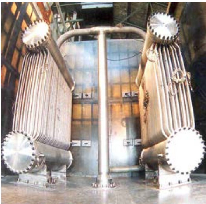
Figura n. 25 - Facility PANTHERS: Passive Containment Condenser
