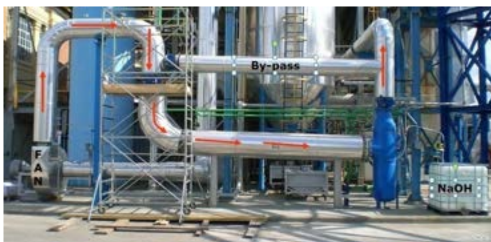
Figure 4 Condenser and neutralization system
