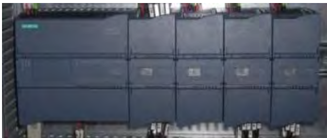
Figura 31. PLC Siemens S7-1200
