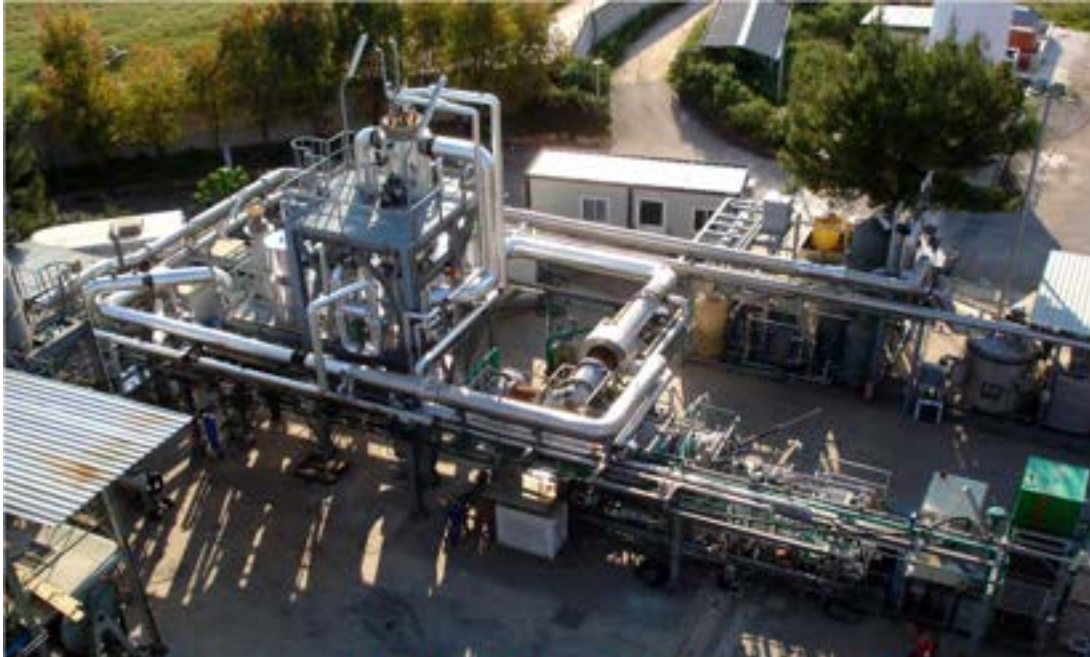
Build-up, in Sulcis area, of a 50 MW th demonstration oxycombustion unit working ant 10 bar pressure
