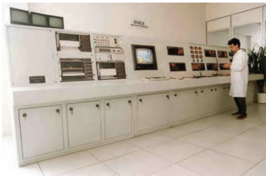
Figure 6 – Test Facility control room
