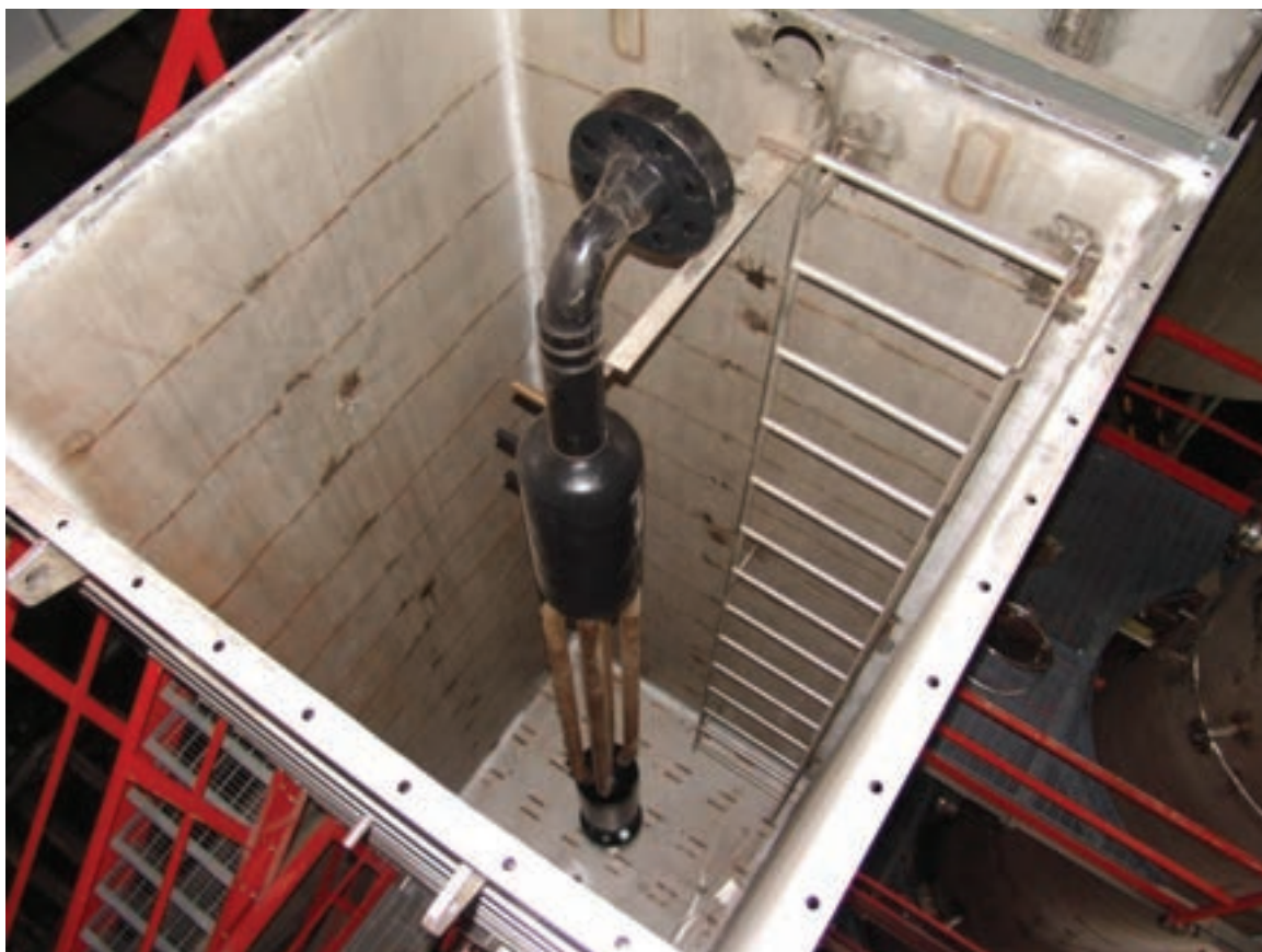
Figure 5 – SPES 3 condenser pool with condenser: inside view
