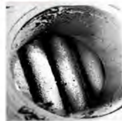
Slag deposit in heat exchanger
