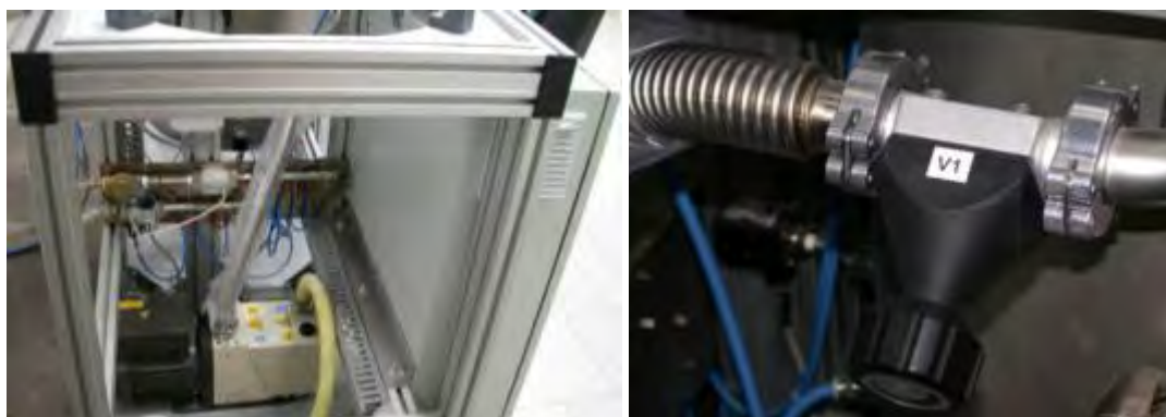
Figure 4: Vacuum pump pipe connections
