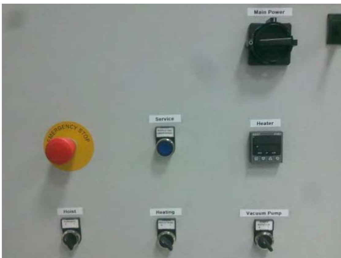
Figure 11: Electrical main panel
