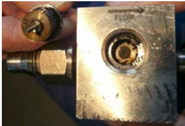
Figure 12: “black mud” after shaft assembly removal
