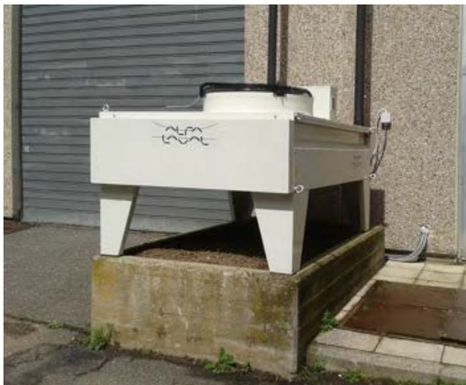
Figura 15. Dry Cooler Alfa Laval
