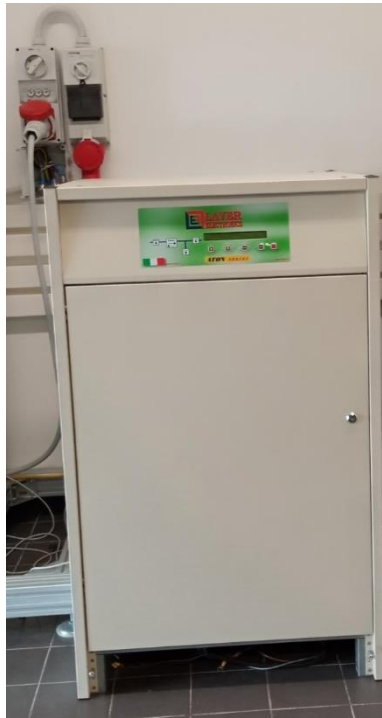
Figura 3: Power Energy Interface
